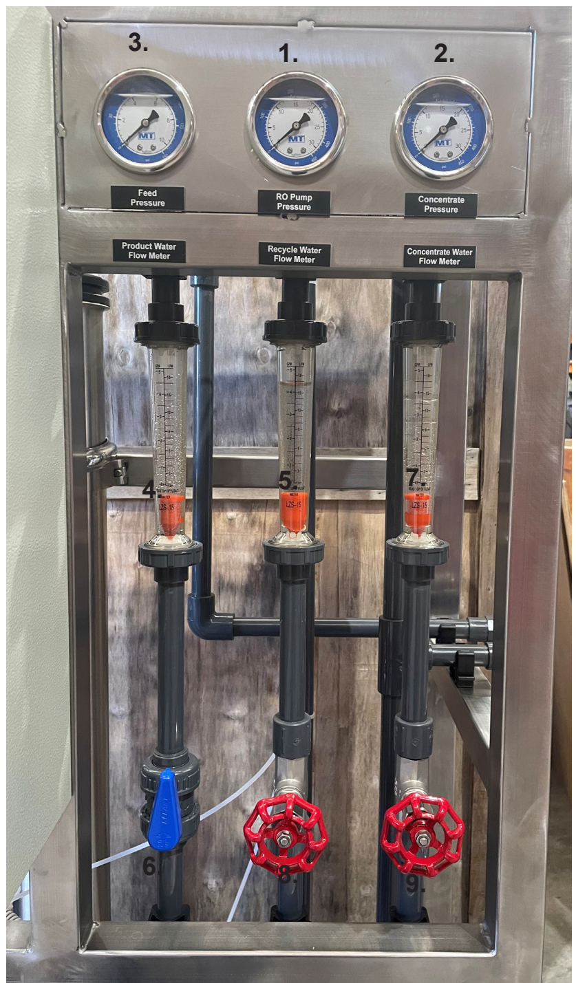
Picture 5.2 WERO4 Flow meters and pressure gauges
